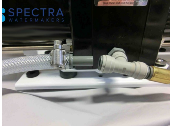
From Feed pump to Clark Pump
