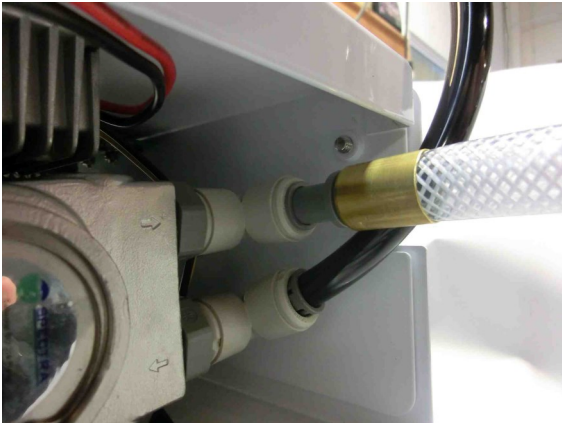
Pump out on Feed Pump Module
