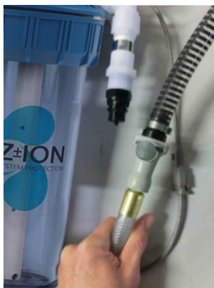
Removing hose to sea strainer from the “to strainer” pigtail.
