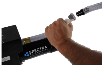
*Connecting brine discharge service hose at quick disconnect
