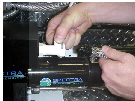
Attaching brine discharge service hose
