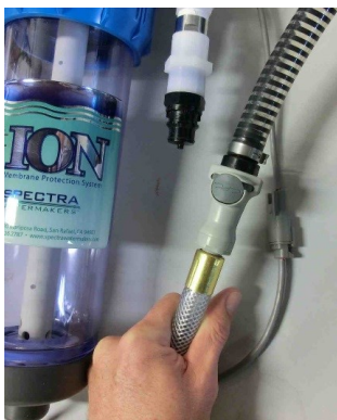
Removing hose to sea strainer from the “to strainer” pigtail.
