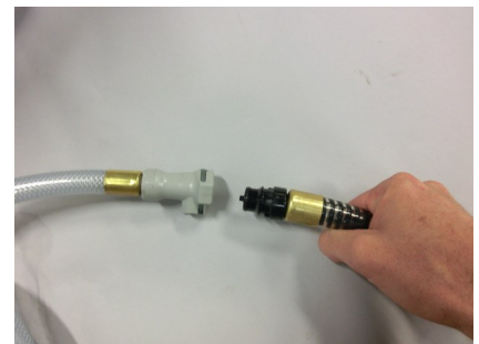
Attaching intake service hose to the hose connecting to the sea strainer.
