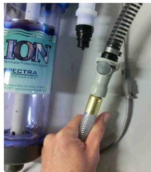
Removing hose to sea strainer from the "to strainer" pigtail.
