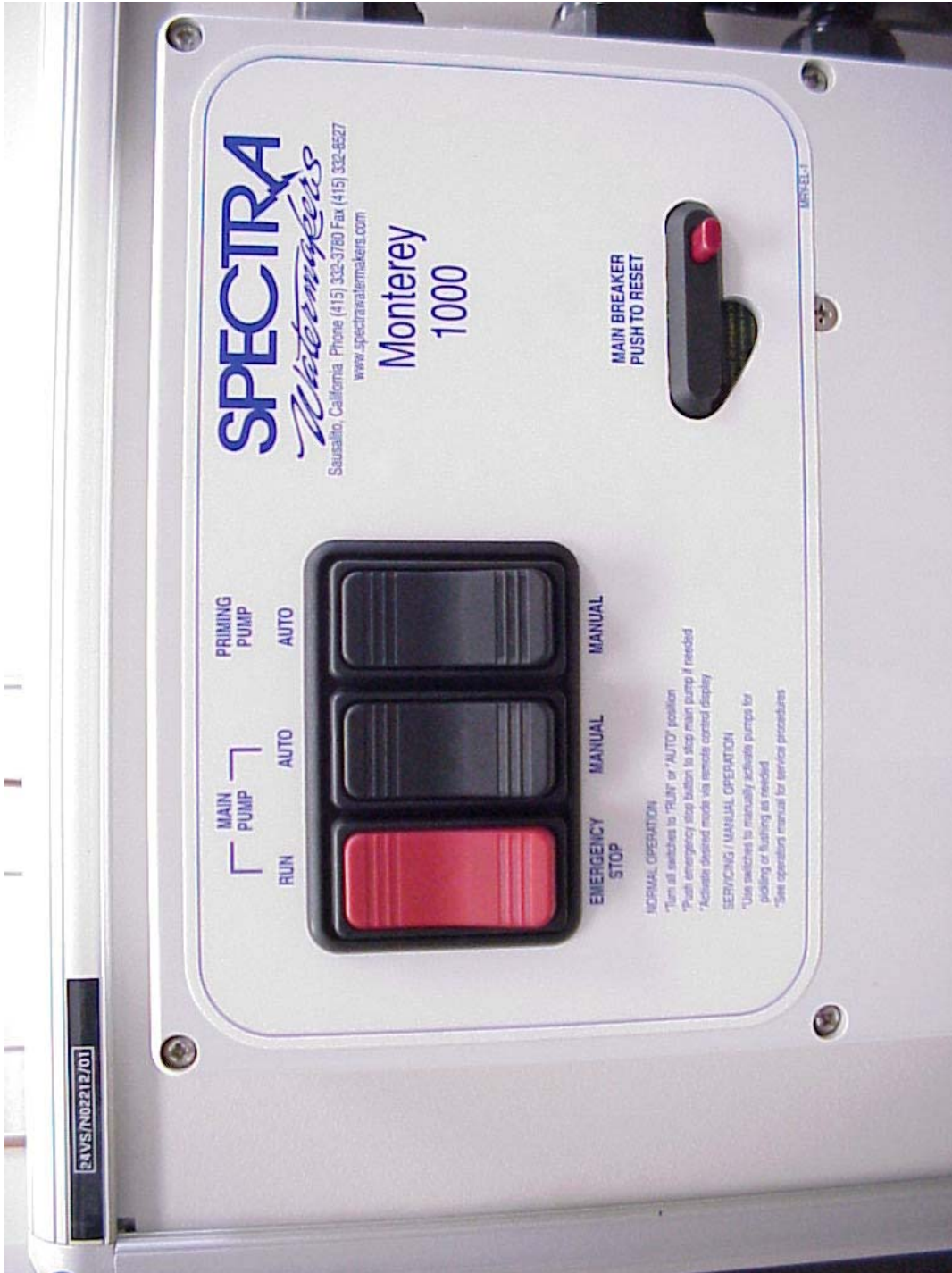
Monterey DC Main Breaker, Emergency Stop & Manual Control Switches
